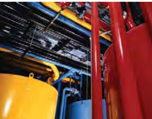
Compressed Air Systems
